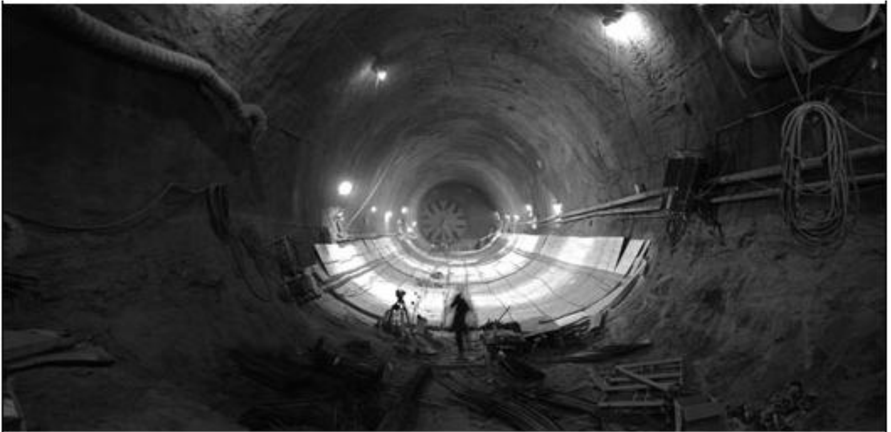
Photo of Beacon Hill Tunnel under construction by Sound Transit Photographer in Residence Peter deLory
